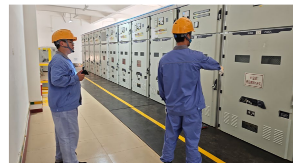
Simulate on-site switching operations under severe weather conditions prior to typhoons
