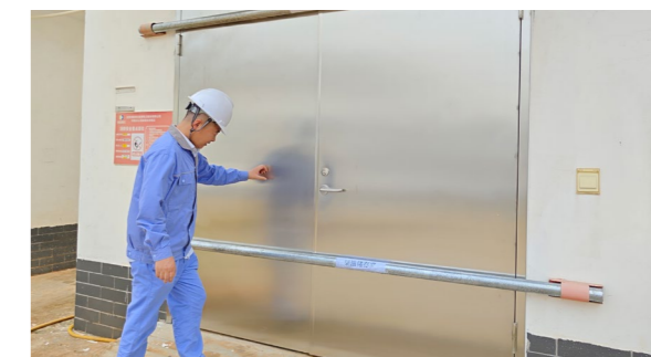
Reinforce gates in advance
